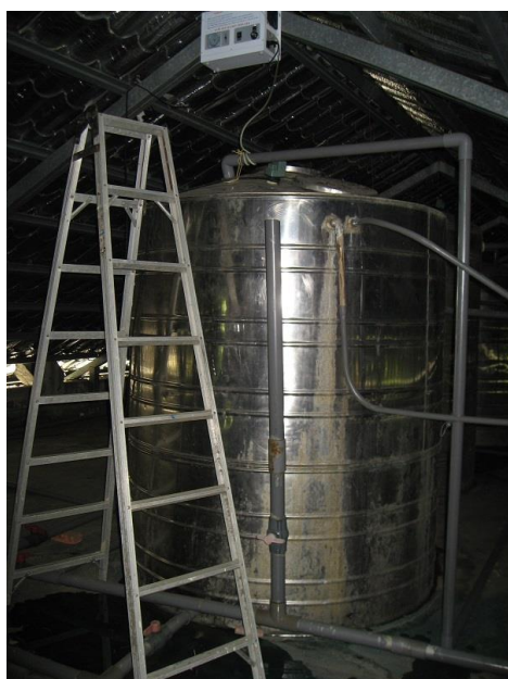
(c)臭氧導入水塔
